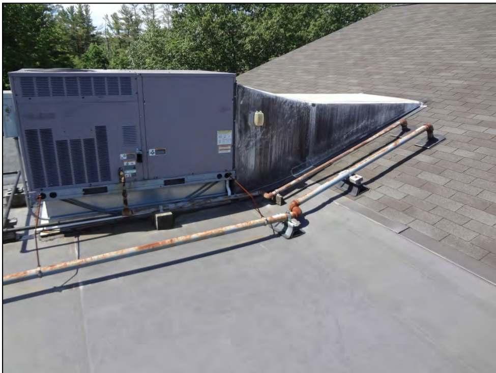
Gas piping needs repainting and supports.
