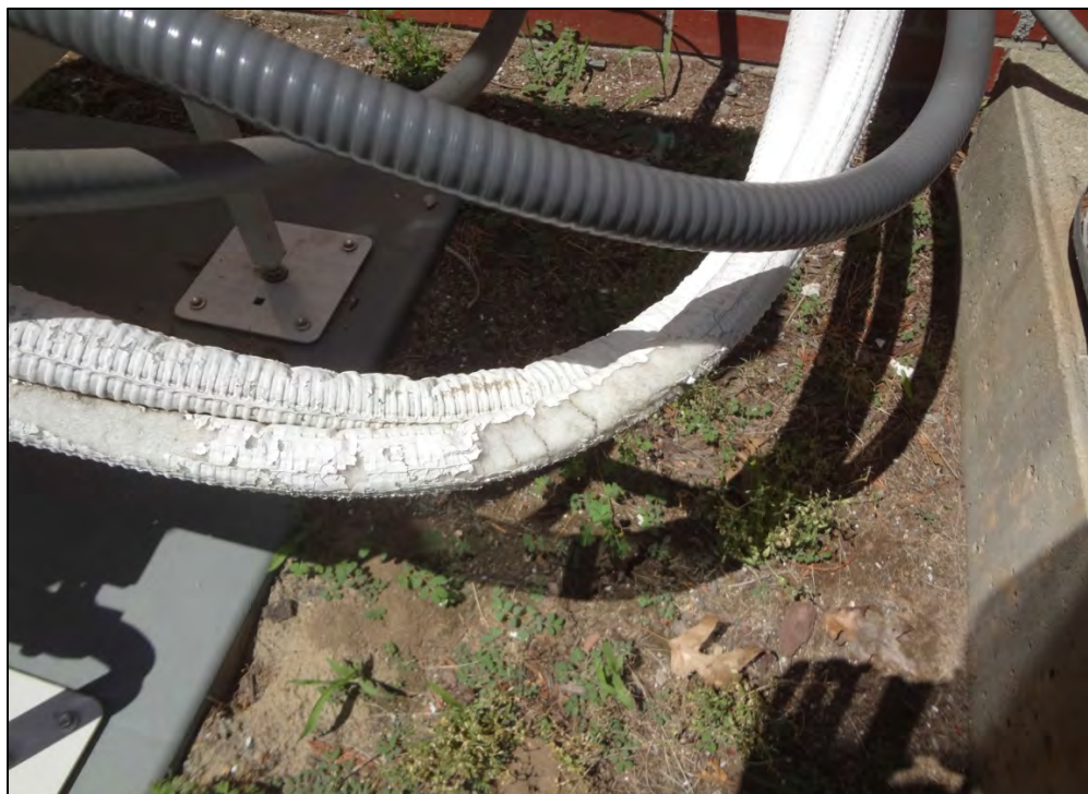
Insulation on cooling lines needing replacement.
