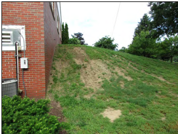
Sparse grass-cover on north side slope.
