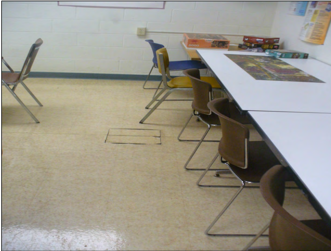
Sheet vinyl in break room needs replacement.
